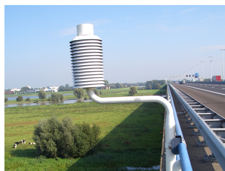
Figure 3: Air Temperature sensor, next to the road.
